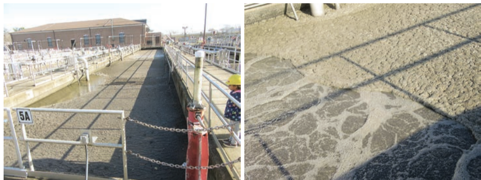
This wastewater is undergoing secondary or biological treatment using bacteria.
