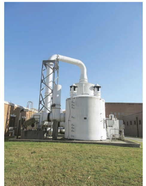
A biotower, odor control technology.
